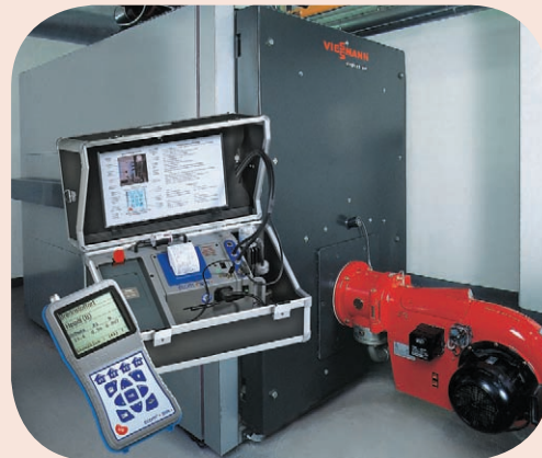
J2KN at Viessmann oil boiler
