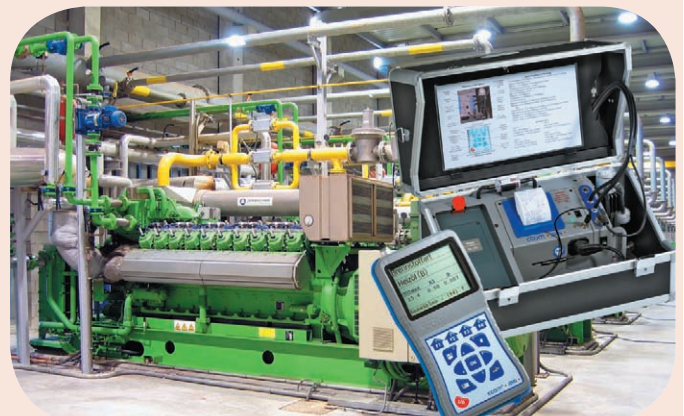
J2KN at Jenbacher combined heating and power station
